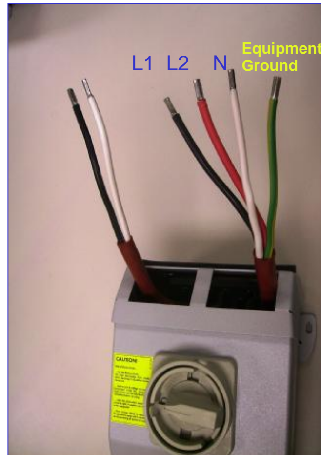
New Disconnect : There is a dedicated Equipment Ground wire to the Inverter
