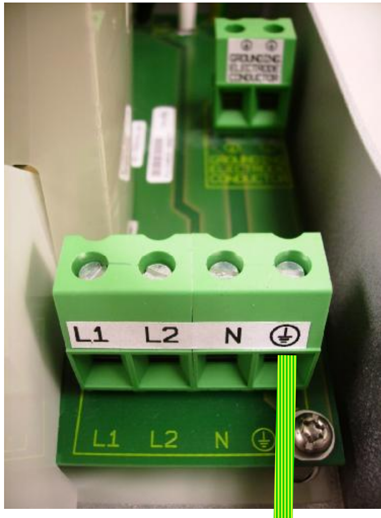
Equipment Ground from the AC distribution panel
