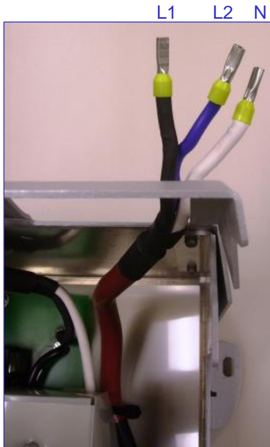
Old Disconnect : No Equipment Ground Wire; Eq.Gnd. is transferred mechanically to inverter chassis.
