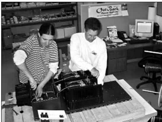
Eric and Dan work together to build a ReadyWatt® integrated, off-grid power center at Energy Outfitters' ETL® certified ReadyWatt® assembly facility in Grants Pass, Oregon.
