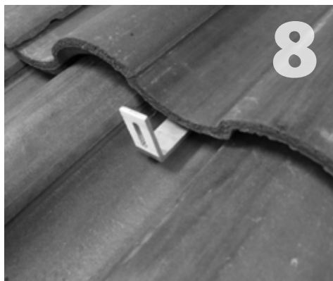
8 Bolt the side-mounted rail of your choice to the hook, using the rail manufacturer's hardware.
