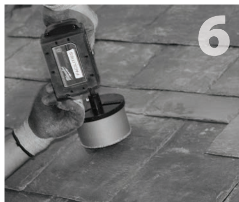
Using a 4" diameter diamond hole saw and the pilot hole drilled in step 3, drill through the existing slate.
