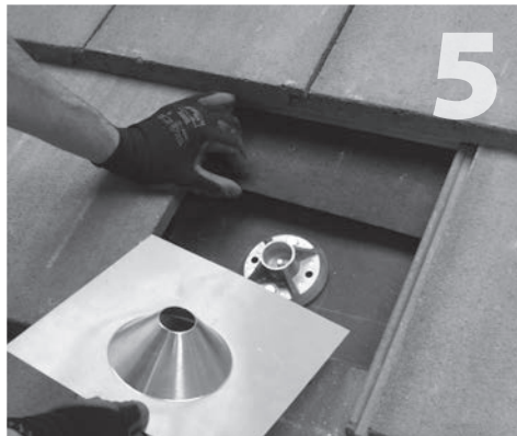
Install subflashing (item 5) in either the lapped paper method explained on this page or the three-course method explained on the next page.
